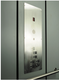
Trapped person presses the emergency call button
